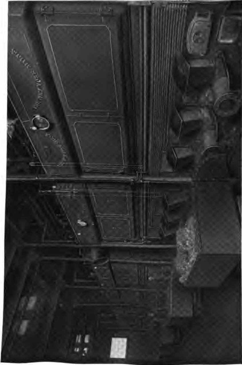
A part of the 4500 H. P. Installation of Heine Standard Boilers equipped with Jones Underfeed Stokers in the Plant of The New York Mills Corp., New York Mills, N. Y.
