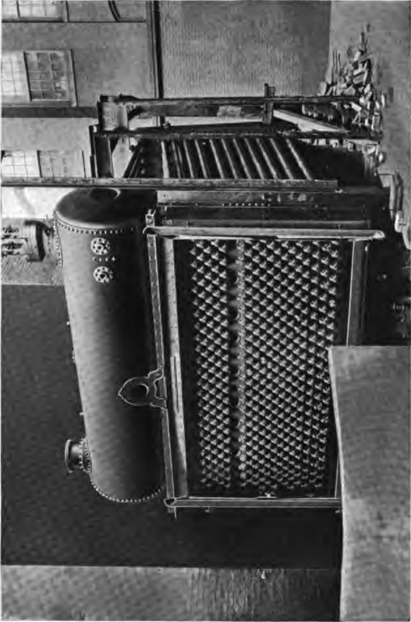
Heine Cross Drum Boiler of 437 H. P., in course of erection at the plant of the Phoenix Underwear Co., Little Falls, N. Y.
