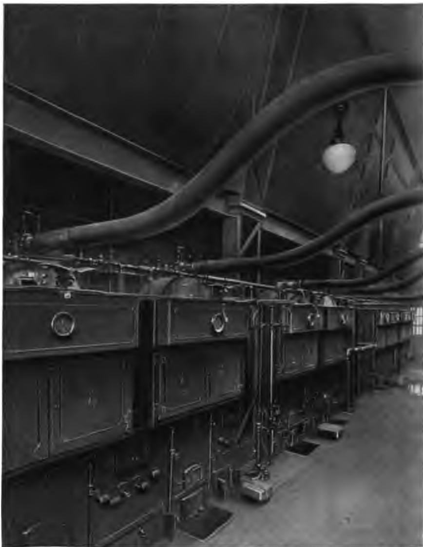
Installation of 2500 H. P. of Heine Standard Boilers in the Ridgewood Pumping Station, Brooklyn, N. Y.
