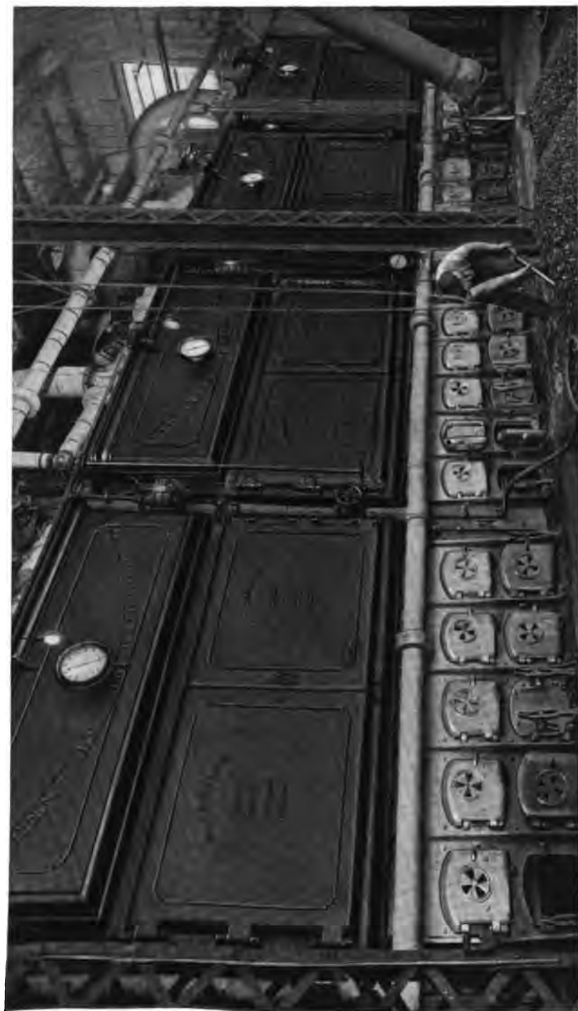
2000 H. P. installation of Heine Standard Boilers in the Broad Street Station of the Pennsylvania Railroad, Philadelphia, Pa. This company operates 10,000 H. P. of Heine Boilers.
