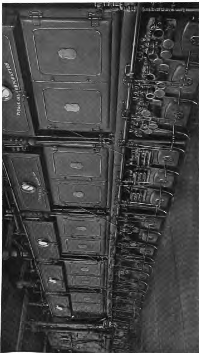
A part of 3388 H. P. installation of Heine Boilers in the Sand Springs, Okla. plant of the Pierce Oil Corporation. This company operates 5650 H. P. of Heine Boilers.
