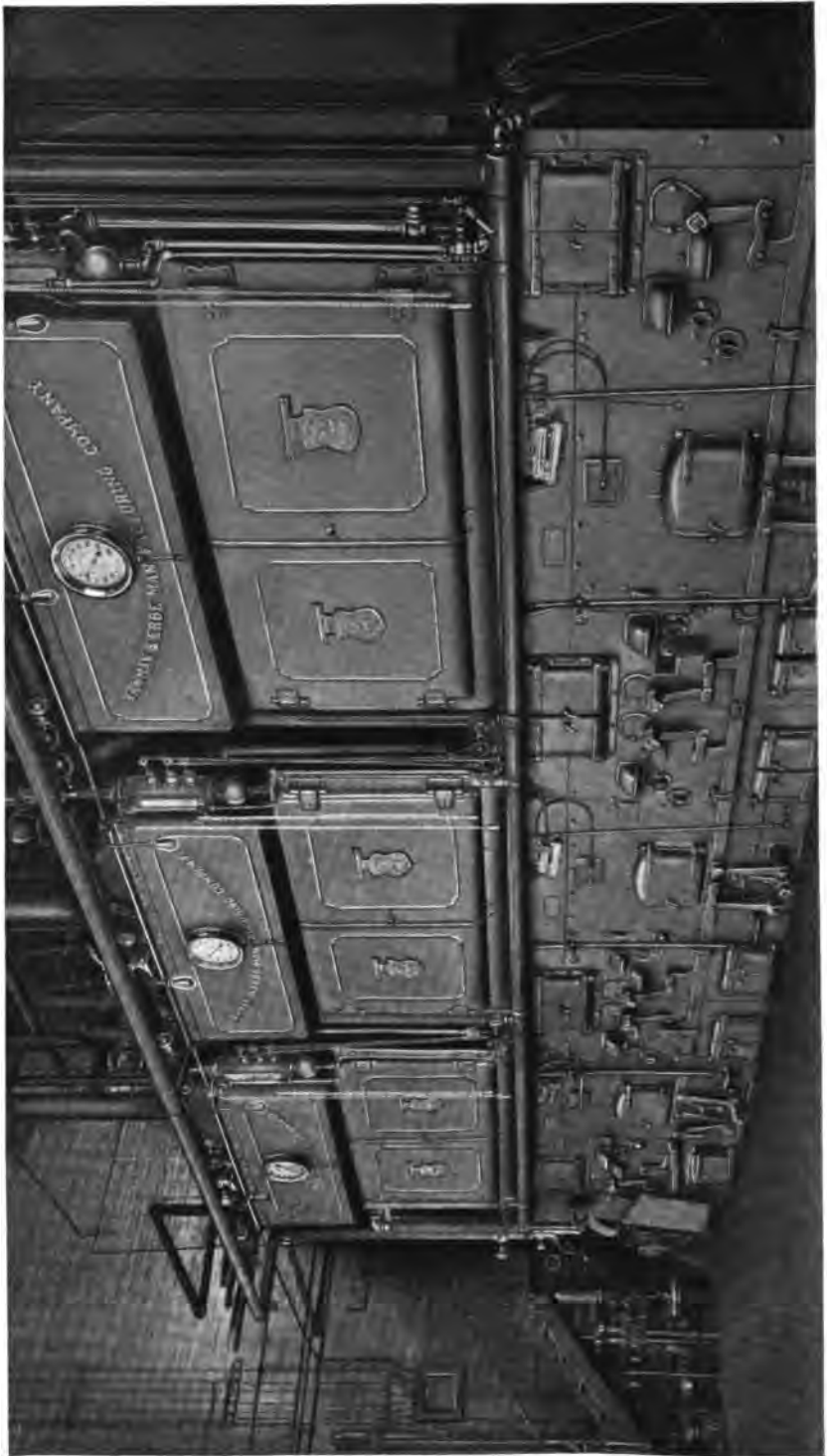
Three 250 H. P. Heine Standard Boilers set over Murphy Stokers in the Plant of Yawman & Erbe Co., Rochester, N. Y.
