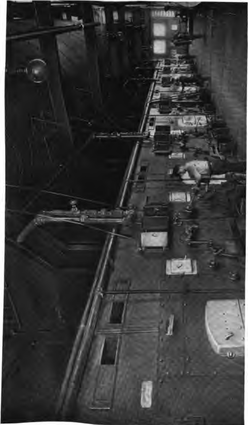
A part of Boiler Room No. 2 of the Federal Sugar Refining Co., Yonkers, N. Y. 7606 H. P. of Heine Standard Boilers, with Murphy Stokers.
