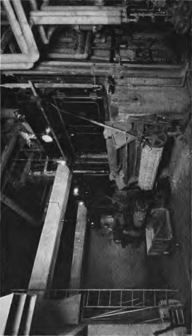
Three 308 H. P. Heine Standard Boilers equipped with Green Chain Grate Stokers installed in the Kimball Building, Chicago, Ill.
