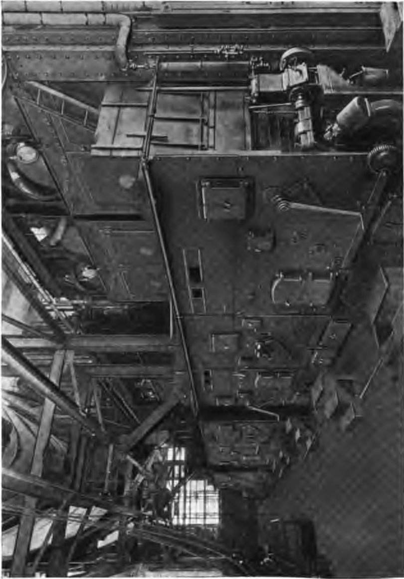
3000 H. P. of Heine Standard Boilers equipped with Heine Superheaters and Murphy Stokers in the Plant of the New York Air Brake Co., Watertown, N. Y.
