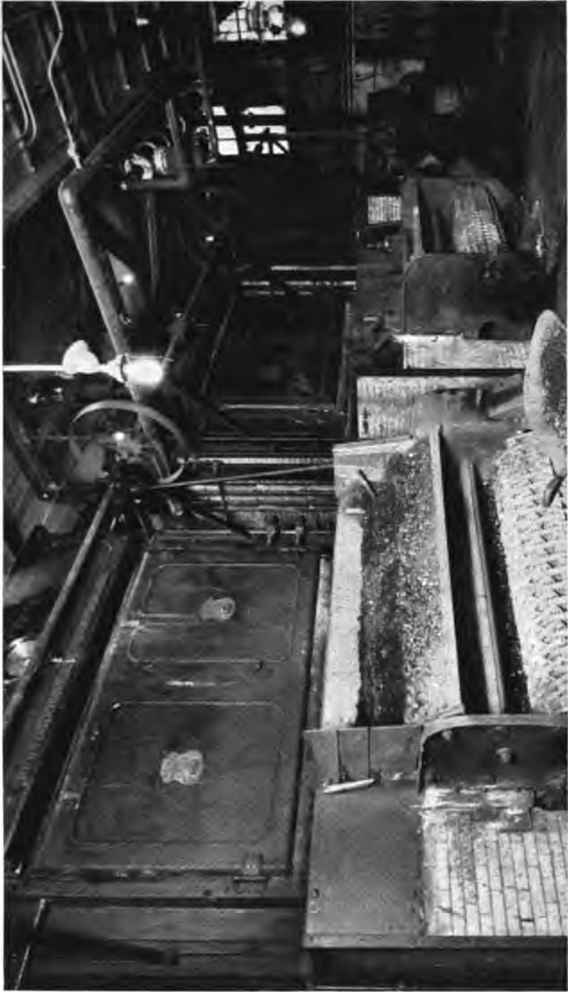
Three 360 H. P. Heine Standard Boilers equipped with Laclede-Christy Chain Grate Stokers installed in the Mercy Hospital, Chicago, Ill.
