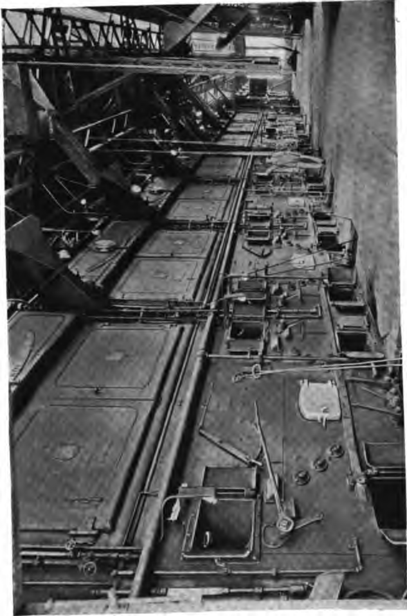
Part of 1600 H. P. Installation of Heine Standard Boilers set over Murphy Stokers in the United States Navy Yard, Norfolk, Va. 1500 Additional H. P. of Heine Standard Boilers are Installed in the Naval Hospital in this Yard.
