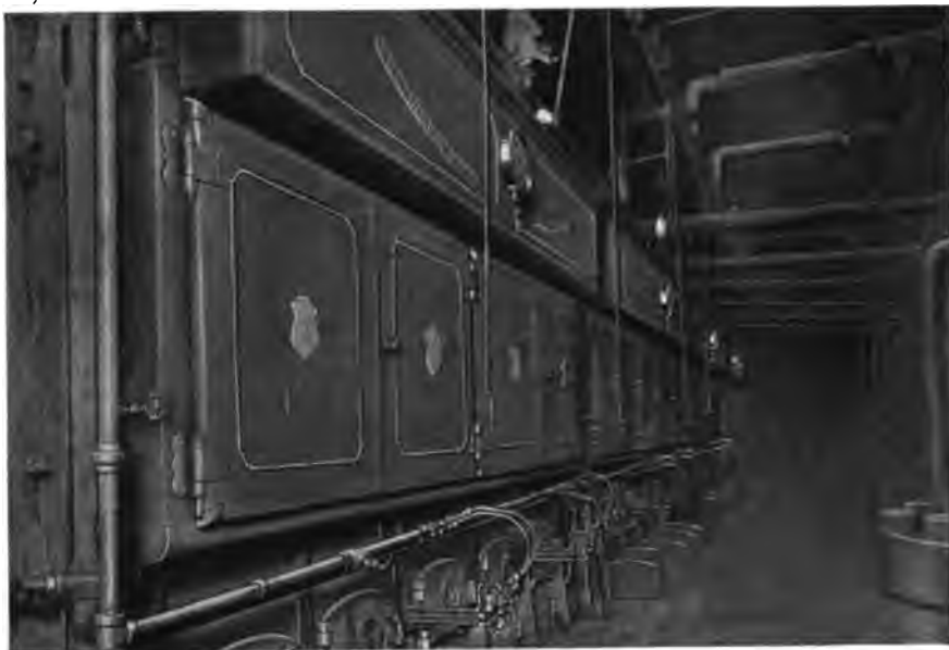
West Side Station, Denver Gas & Electric Co., Denver, Colo. Part of 10,000 H. P. of Heine Standard Boilers and Heine Superheaters.
