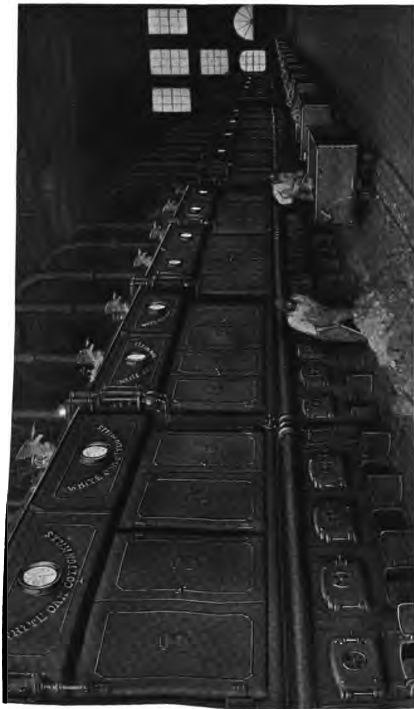
White Oak Cotton Mills of the Proximity Mfg. Co., Greensboro, N. C., containing 6300 H. P. of Heine Standard Boilers. This company operates 9050 H. P. of Heine Boilers.
