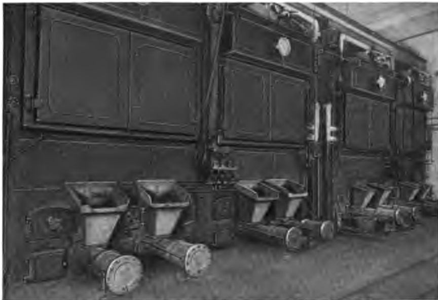
Four 315 H. P. Heine Standard Boilers set over Jones Underfeed Stokers in the Hamilton County Court House, Cincinnati, Ohio.
