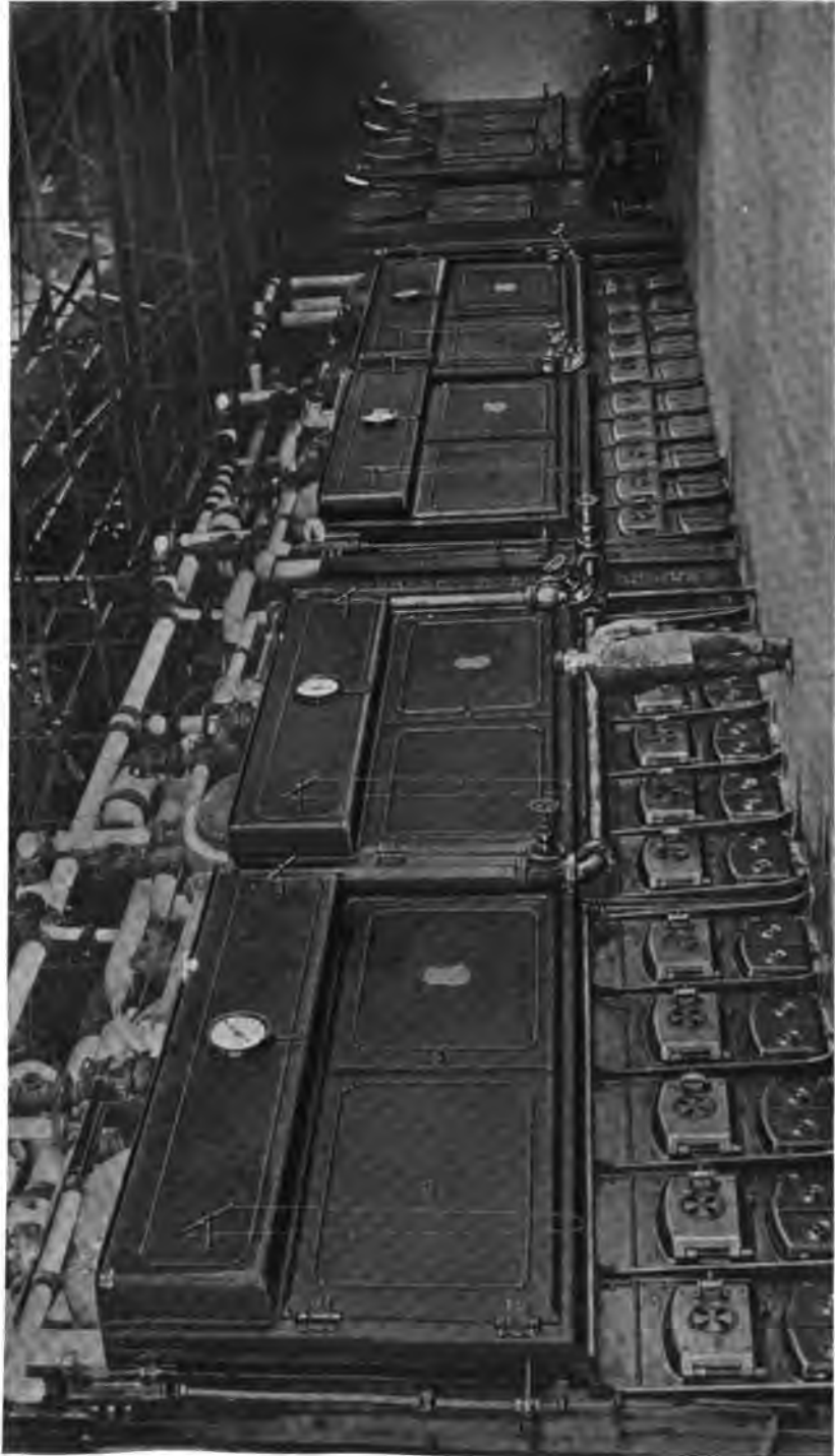
2000 H. P. Heine Standard Boilers in the Sumitomo Besshi Mines, Japan.
