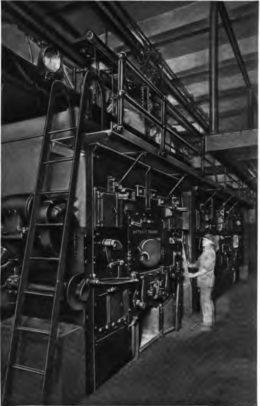
Three Heine Standard Boilers, in the American Express Co. Building, New York City, set over Detroit Stokers.
