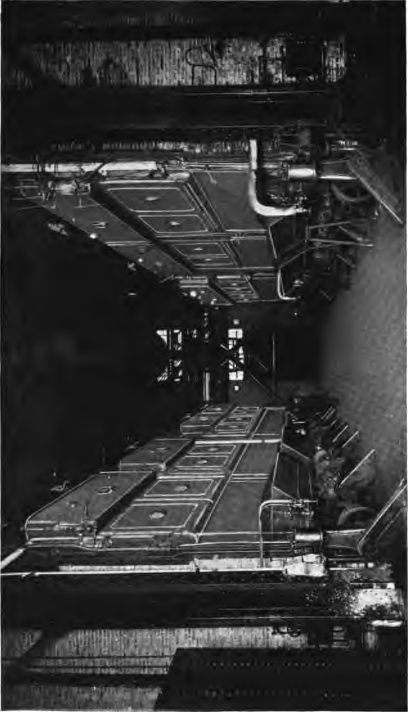
4200 H. P. Installation of Heine Standard Boilers and Heine Superheaters set over Taylor Stokers in the Plant of the Studebaker Corp., South Bend, Ind.
