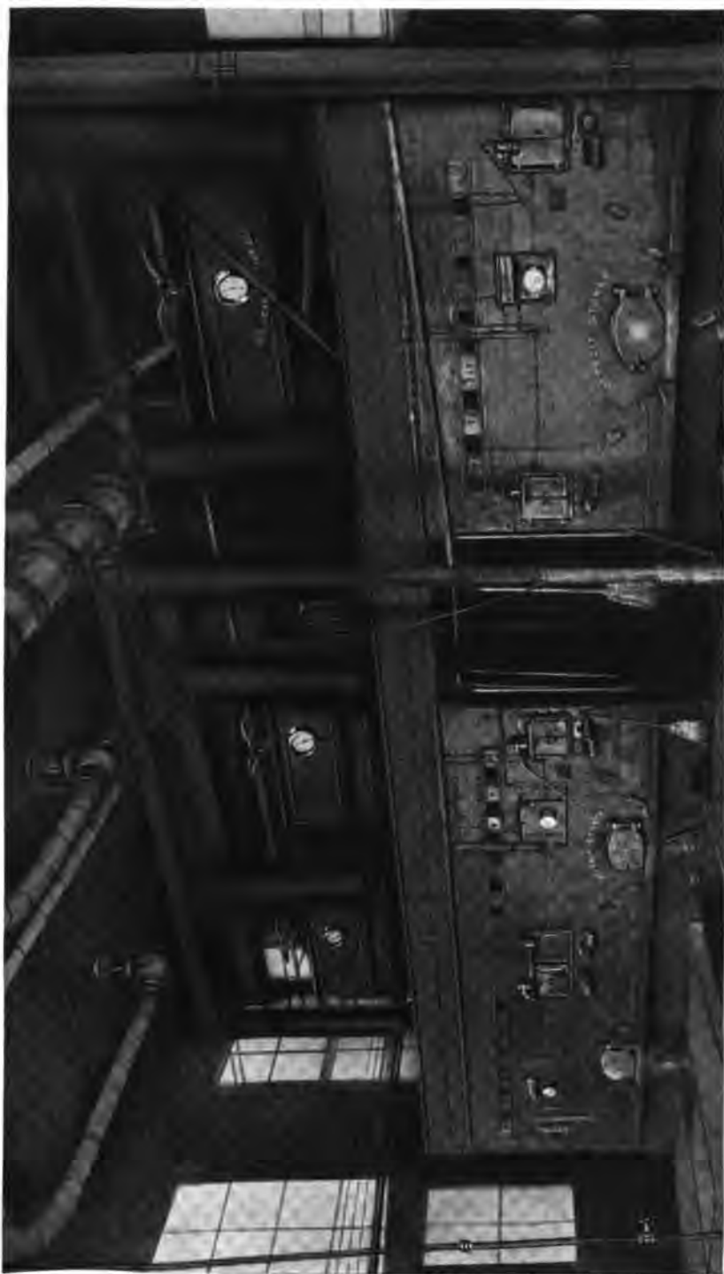
Three 330 H. P. Heine Standard Boilers set over Detroit Stokers in the Plant of Joseph Joseph & Bros. Co., Cincinnati, Ohio.
