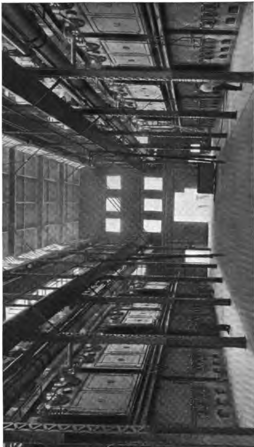
Sixteen 518 H. P. Heine Standard Boilers, equipped with Oil Burners, installed in a large Oil Refinery. This is part of the same H. P. of Heine Standard Boilers installed in this plant.
