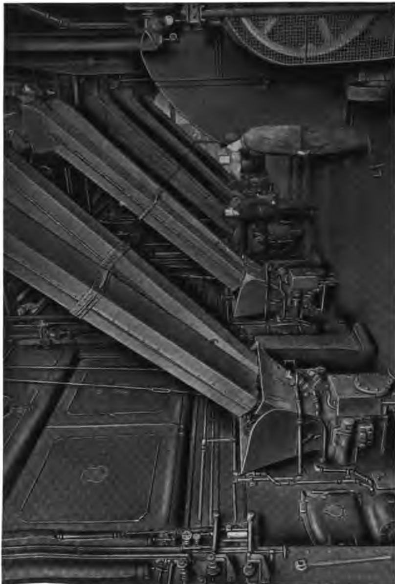
A part of the 2000 H. P. installation of Heine Boilers in the Hecker-Jones-Jewell Milling Co., New York City.
