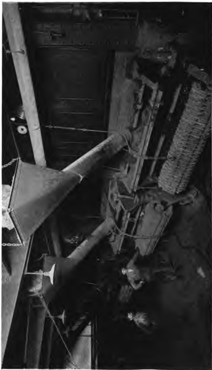
1000 H. P. Heine Boiler installation in the Robey Street Terminal of the Baltimore & Ohio Railroad Co., Chicago, Ill.
