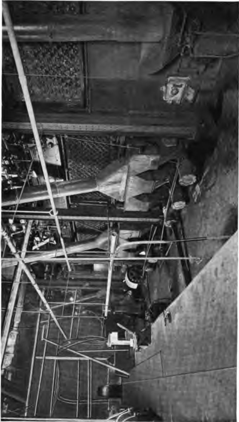
Five 500 H. P. Stoker-fired Boilers. Nearest Boiler equipped with Combustion Engineering Corp. Stoker; remainder with Jones Underfeed Stokers. These Boilers are part of the 5800 H. P. Installation of Heine Standard Boilers at the Pillsbury Flour Mills, Minneapolis, Minn.
