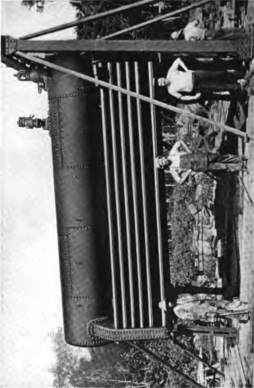
Erecting Heine Standard Boiler for the Caribbean Petroleum Co., Mene Grande, Venezuela.
