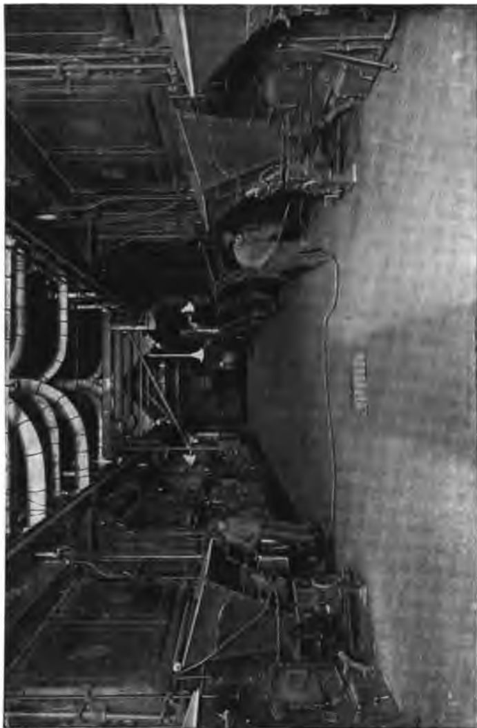
4350 H. P. of Heine Standard Boilers equipped with Combustion Engineering Corp. Type E Stokers, in the Niagara, Lockport & Ontario Power Co., Lyons, N. Y.
