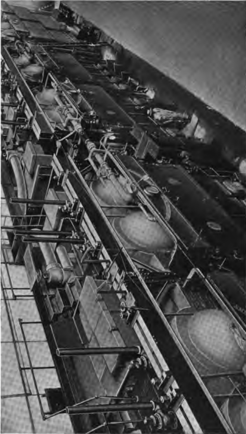
Boiler Room of the Pepperell Mfg. Co., Biddeford, Me., containing 4000 H. P. of Heine Standard Boilers and Heine Superheaters. Boilers in Background are set over Combustion Engineering Type E Stokers.
