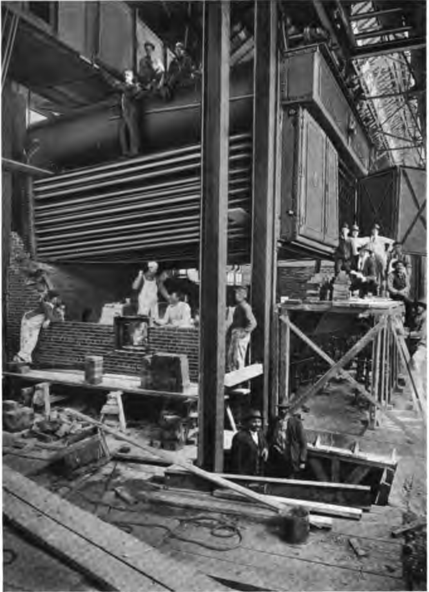
1000 H. P. Heine Standard Boiler in course of erection at the Walter Reed Hospital, Washington, D. C.
