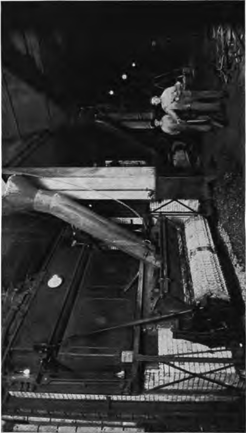
Five 366 H. P. Heine Standard Boilers installed in the Cook County Court House, Chicago, Ill.
