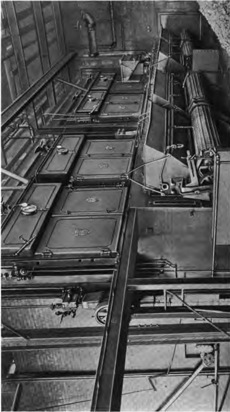
1624 H. P. installation of Heine Standard Boilers set over Green Chain Grate Stokers. General Hospital No. 21 of the United States Army, Aurora, Colo.
