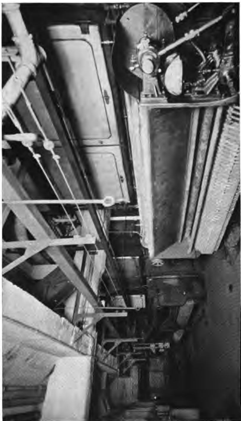
1500 H. P. of Heine Standard Boilers equipped with McKensie Chain Grate Stokers in the Lytton Building, Chicago, Ill.
