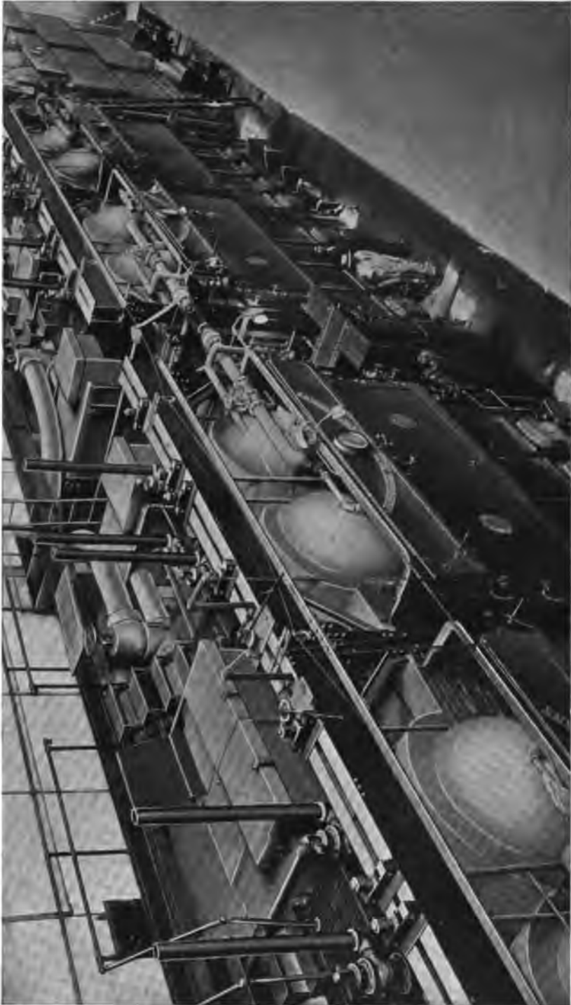
Boiler Room of the Pepperell Mfg. Co., Biddeford, Me., containing 4000 H. P. of Heine Standard Boilers and Heine Superheaters. Boilers in Background are set over Combustion Engineering Type E Stokers.
