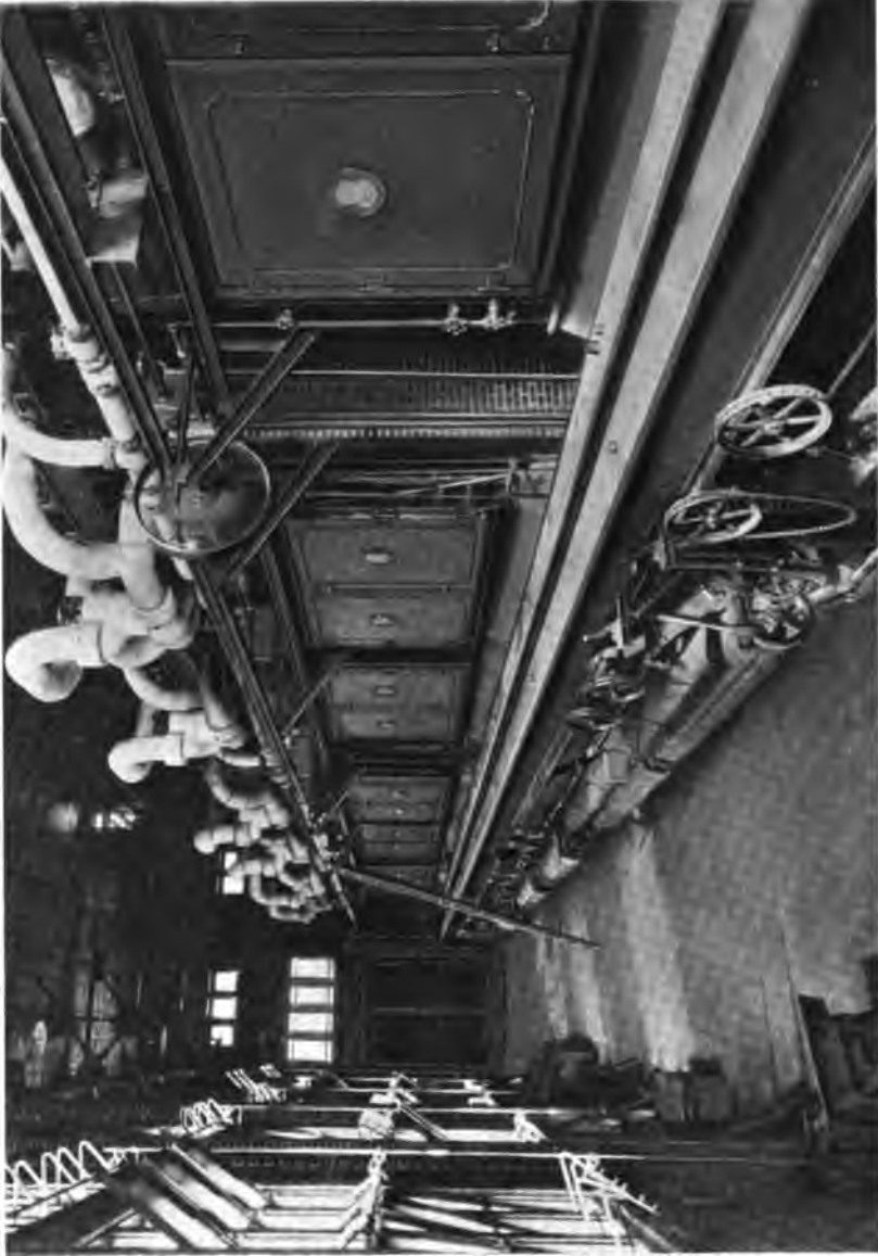
Boiler Room of the River Mines, Mo. Plant of the St. Joseph Lead Co., showing Heine Standard Boilers set over Green Chain Grate Stokers. This Company has installed 7000 H. P. of Heine Boilers.
