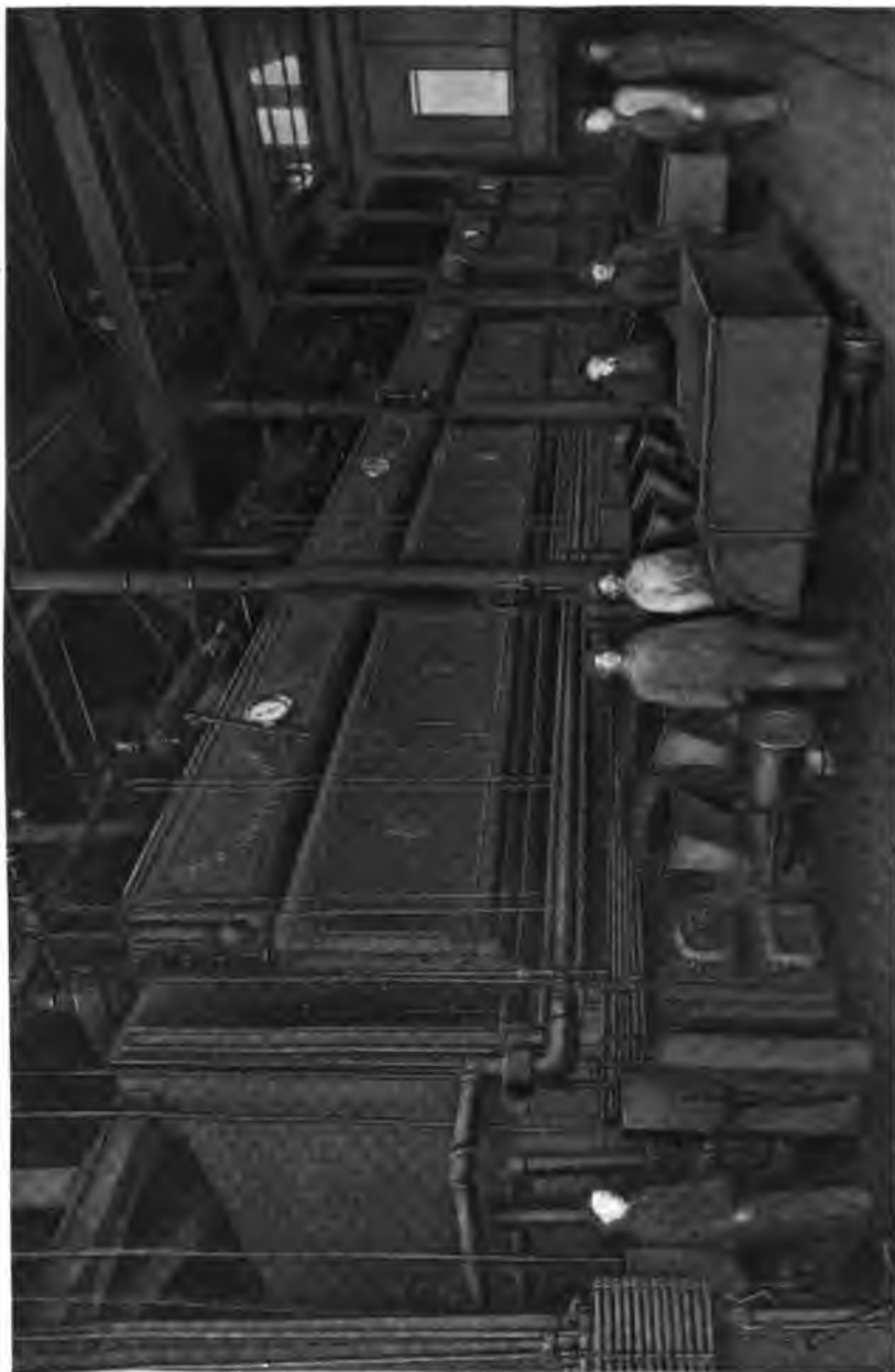
A part of the 4500 H. P. Installation of Heine Standard Boilers set over Jones Underfeed Stokers in the Plant of the New York Mills Corp., New York Mills, N. Y.
