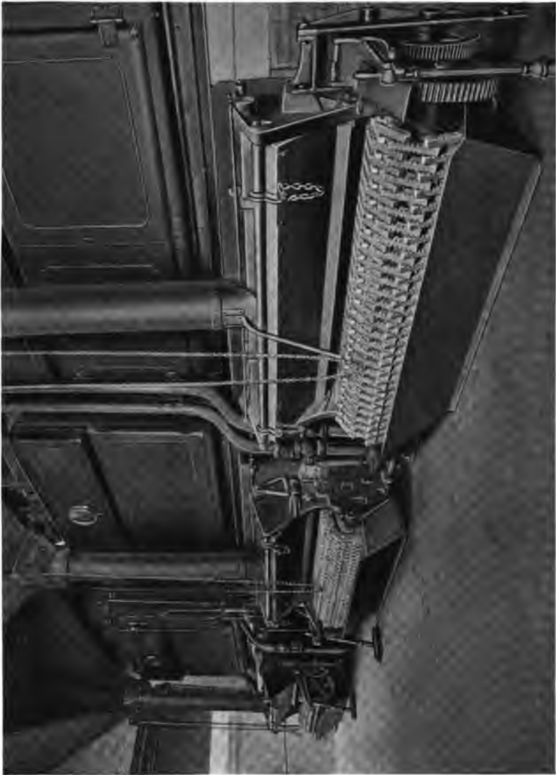
Washington Park Plant of the South Park Commission, Chicago, Ill., containing 1100 H. P. of Heine Standard Boilers set over Green Chain Grate Stokers.
