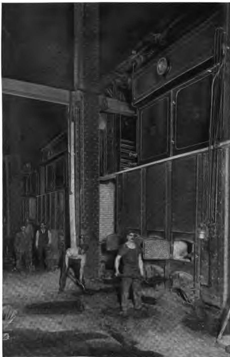
A part of the 3500 H. P. installation of Heine Boilers in the Equitable Office Building, New York City.
