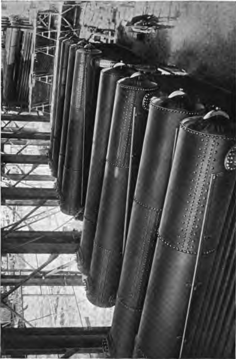
A part of the 6300 H. P. Heine Boiler Installation at the Chino Copper Company, Hurley, New Mexico, in course of Erection.
