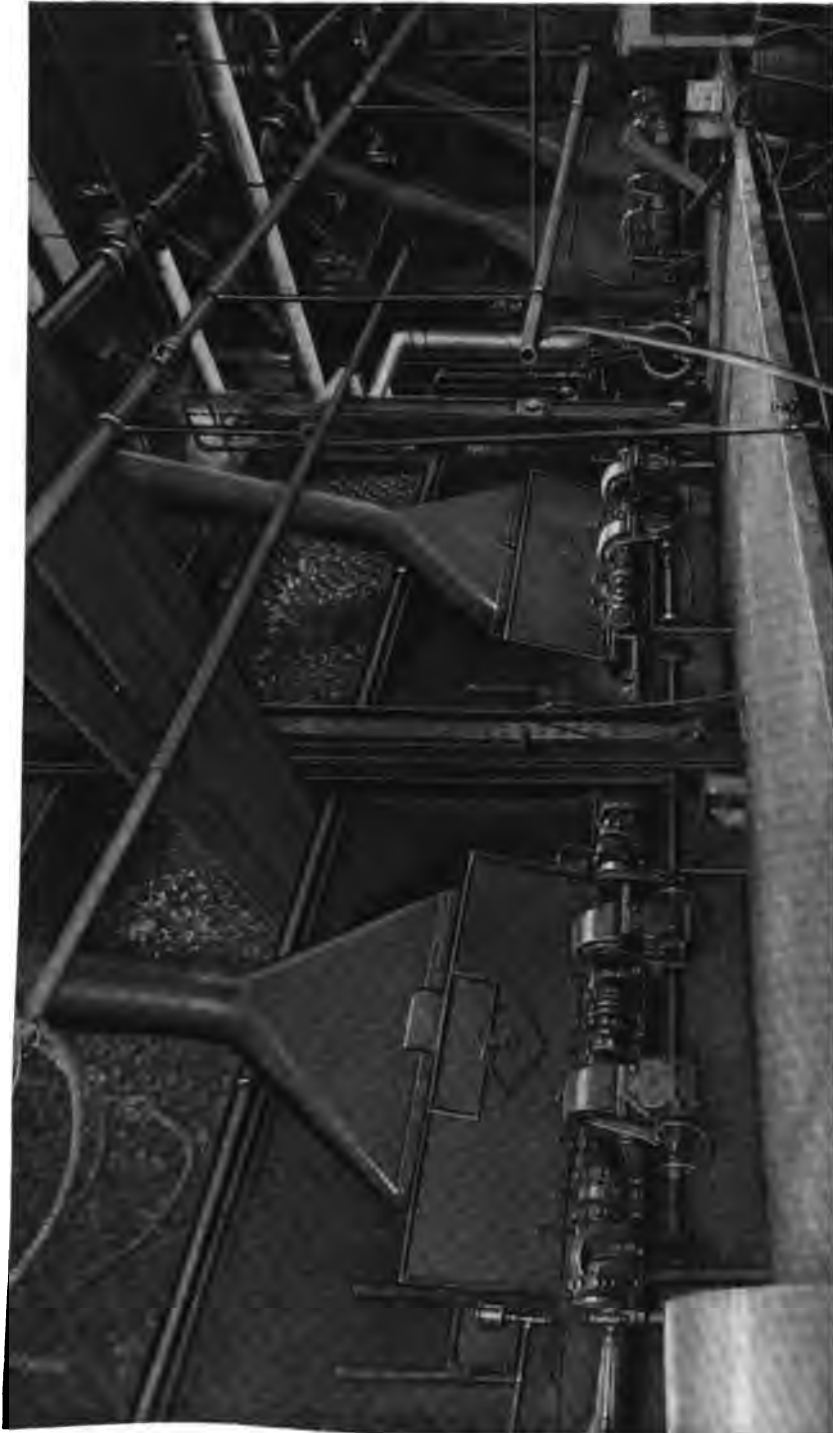
Pillsbury Flour Mills, Minneapolis, Minn. This company has installed 8000 H. P. of Heine Standard Boilers. Boilers shown are set over Sanford Kiley Underfeed Stokers.
