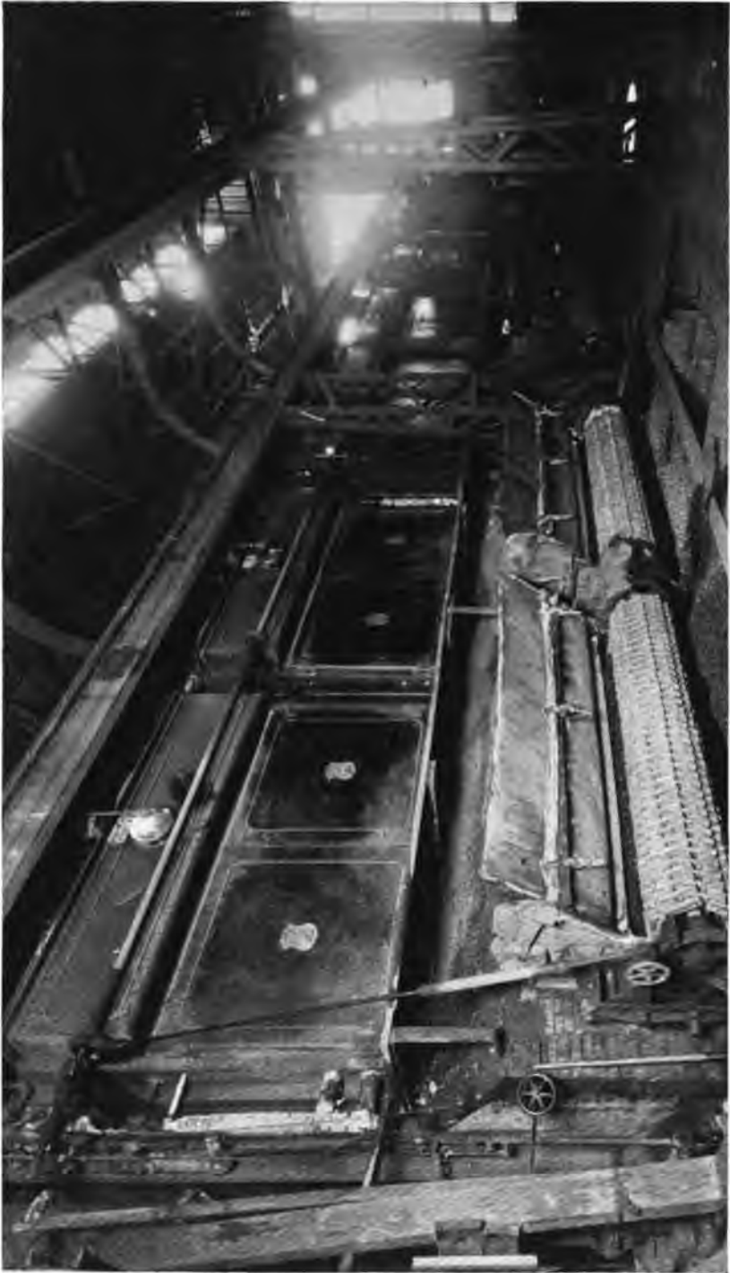
2590 H. P. installation of Heine Standard Boilers equipped with Green Chain Grate Stokers in the Burnside Shops of the Illinois Central Railroad, Chicago, Ill.
