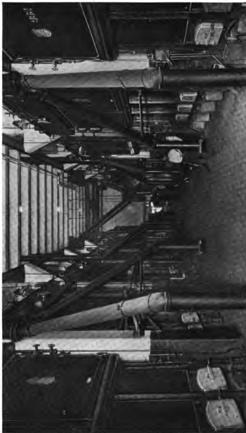
A part of the 8550 H. P. Installation of Heine Standard Boilers and Heine Superheaters in the New York Central Railroad Terminal, New York City. This Company operates 18,000 H. P. of Heine Boilers.
