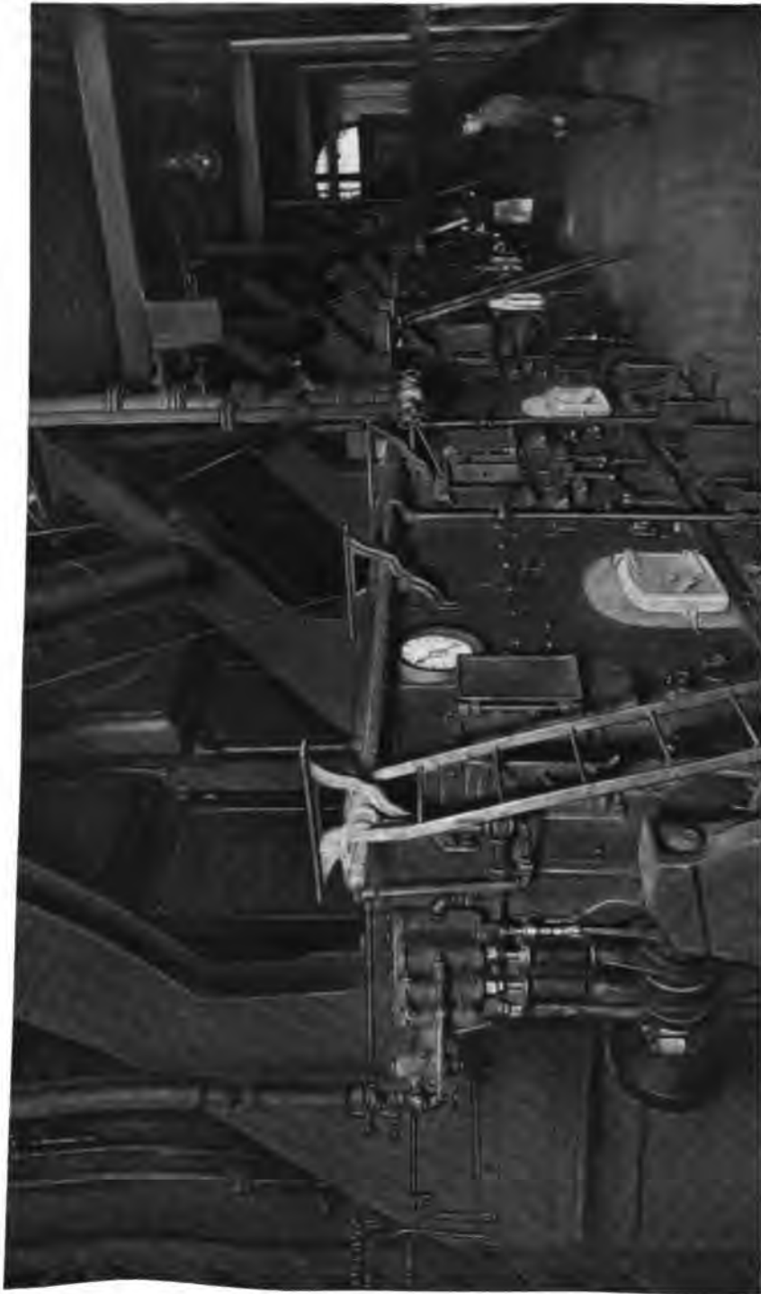
A part of Boiler Room No. 1 of the Federal Sugar Refining Co., Yonkers, N. Y. 7606 H. P. of Heine Standard Boilers, with Murphy Stokers.
