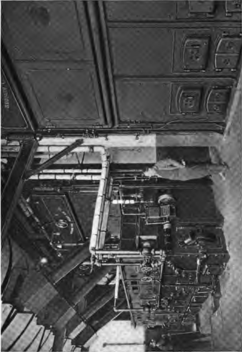
Three 365 H. P. Heine Standard Boilers in the Plant of the Hudson Consumers Ice Co., Hoboken, N. J. Boilers in background set over Murphy Stokers.
