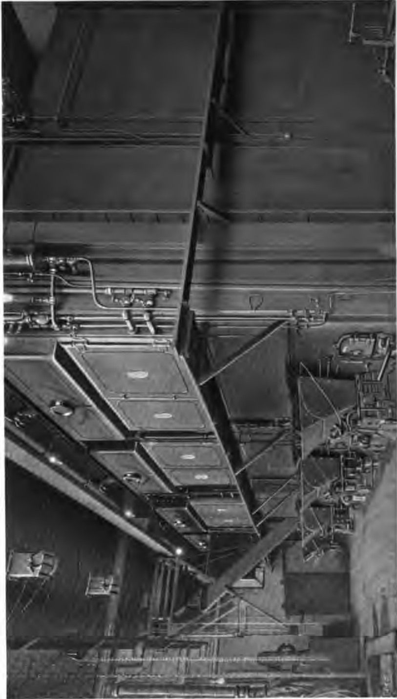
Beck's Run Pumping Station of the South Pittsburgh Water Co., Pittsburgh, Pa. Boilers in this illustration set over Jones Stokers. This company has installed 2600 H. P. of Heine Standard Boilers.
