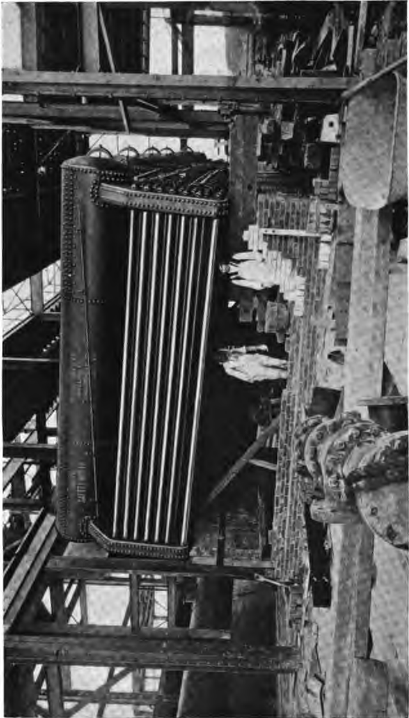
250 H. P. Heine Standard Boiler in course of erection at the Destructor Plant of the Boston Development & Sanitary Co., Spectacle Island, Boston, Mass. The Plant contains 2000 H. P. of Heine Standard Boilers.
