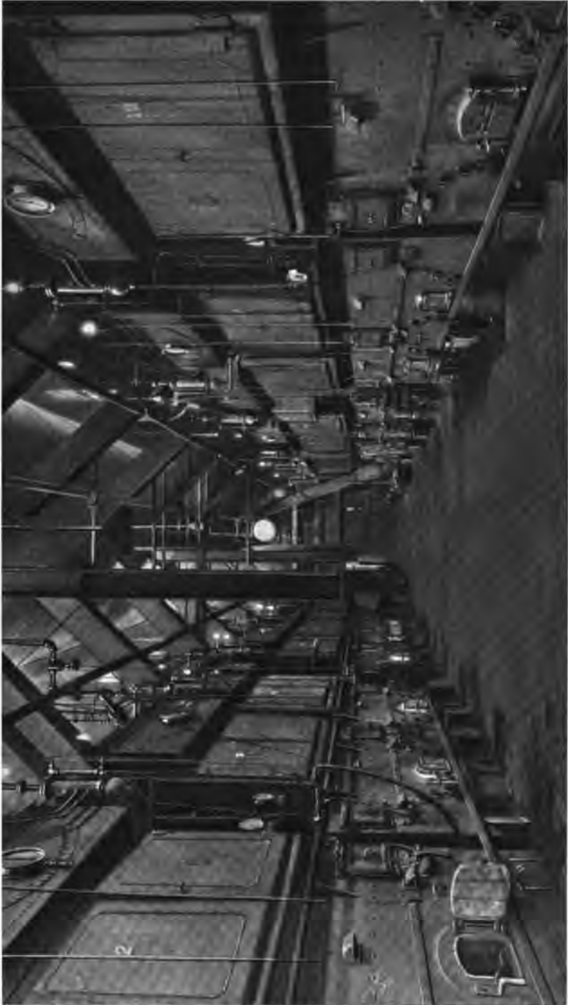
A part of twenty-four 316 H. P. Heine Boilers in the plant of the Champion Fibre Co., Canton, N. C.
