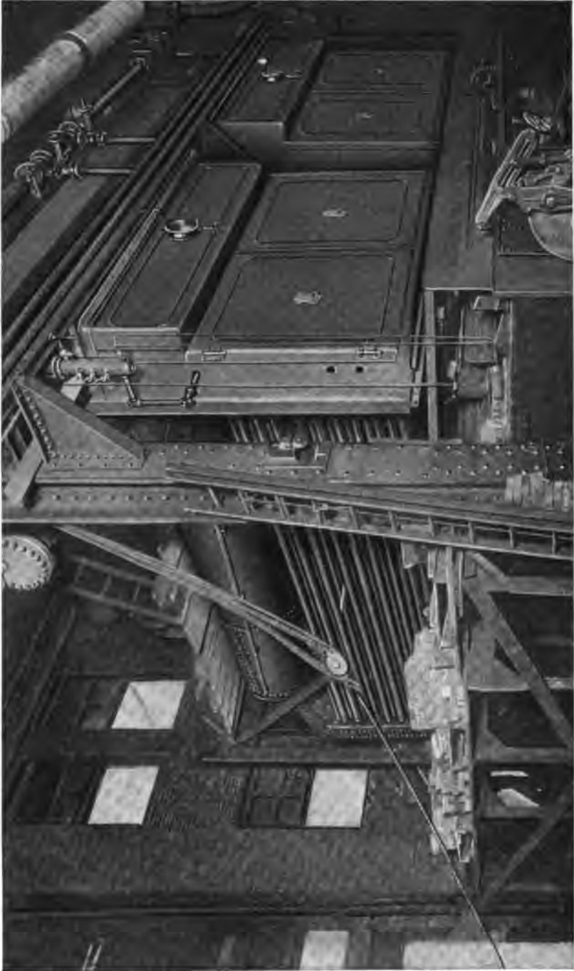
Erecting Two 607 H. P. Heine Standard Boilers in the Pittsburgh, Pa. Plant of the H. J. Heinz Co. This Plant contains 5500 H. P. of Heine Standard Boilers. The Company has Installed in its Subsidiaries 9250 H. P. of Heine Standard Boilers.
