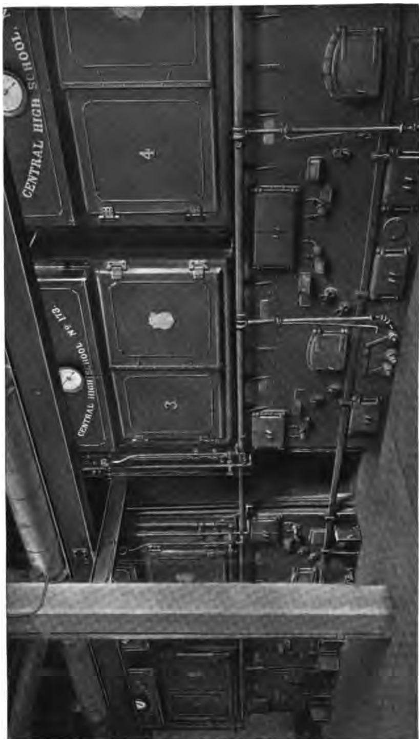
Four 306 H. P. Heine Standard Boilers installed in the Central High School, Washington, D. C.
