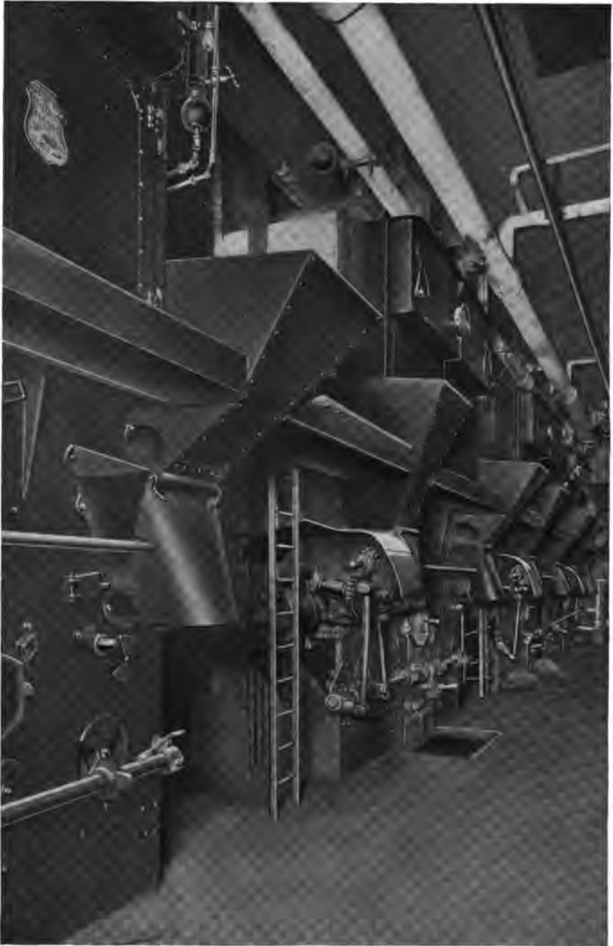
1400 H. P. of Heine Standard Boilers equipped with Murphy Stokers, in the Fifth Avenue Building, New York City.
