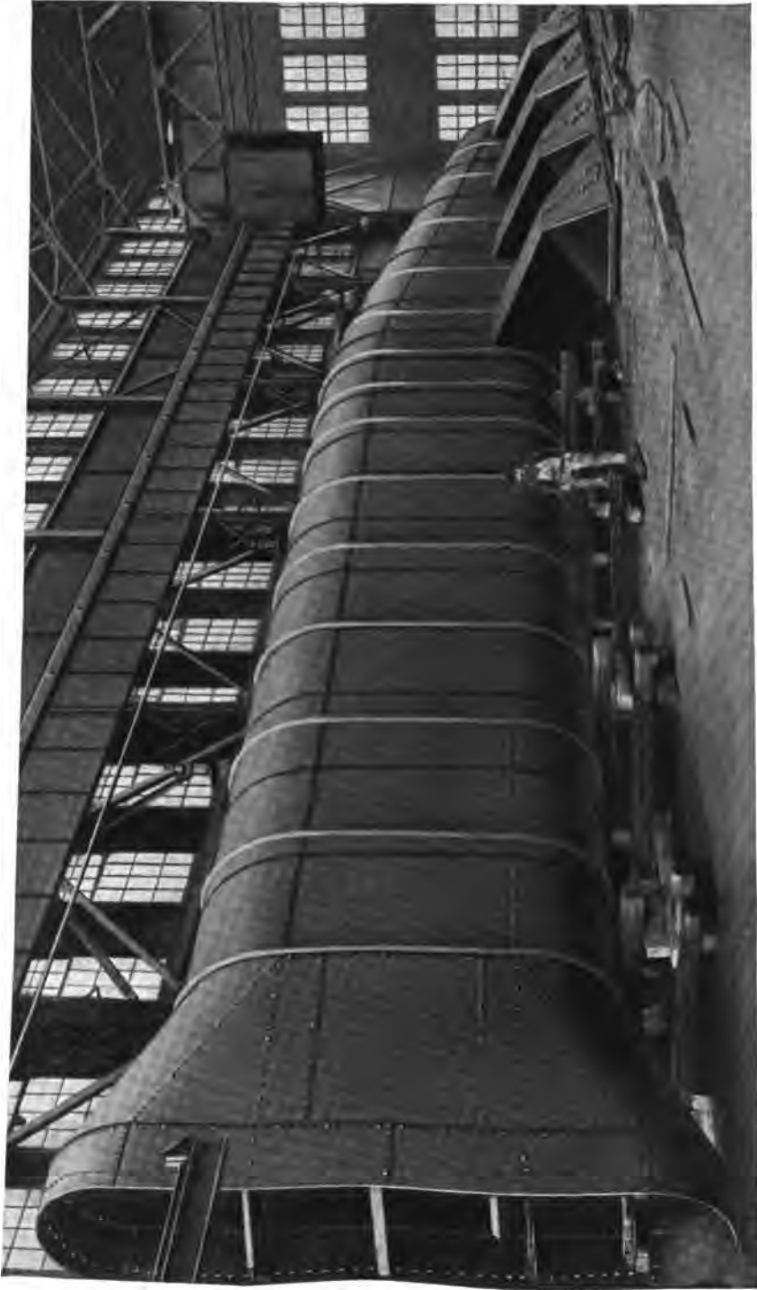
Breeching built for the Norfolk Navy Yard, Norfolk, Va., in which are installed 1600 H. P. of Heine Standard Boilers.
