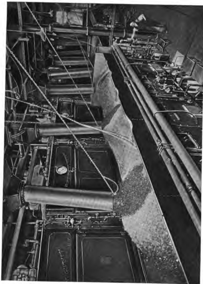
2300 H. P. Installation of Heine Standard Boilers set over Murphy Stokers in the Plant of The Ebling Brewing Co., New York, N. Y.
