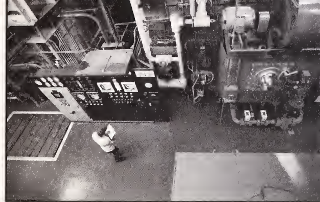
DURING A DAILY ROUTINE, Pat McDiffett, facilities and power plant worker, reads and records gages on a boiler. — Photo by Drew Rose
