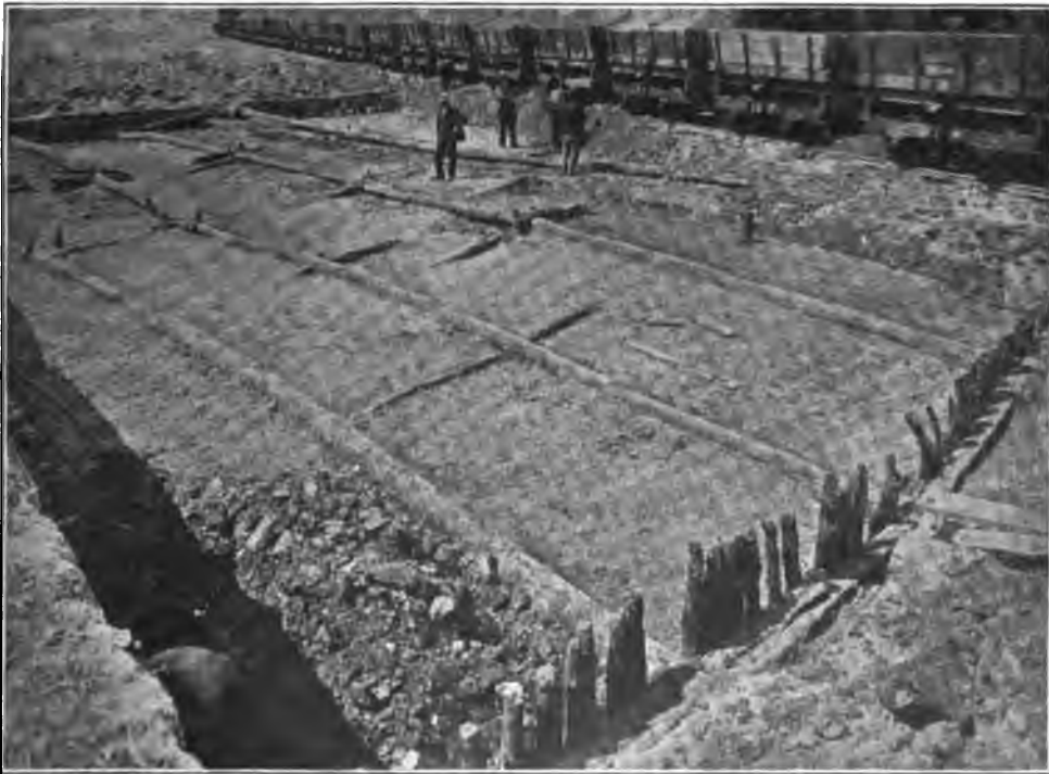
CONSTRUCTION OF THE PILE WORK IN THE ROMAN STRUCTURE AT ZEEBRUGGE [FIG. 2]
