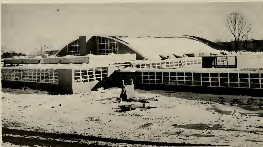
Pictured above is a back view of the unfinished gym. The snow, covering the building, was one reason for the delay in construction.
