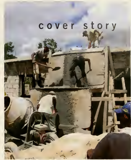
Workers construct a roof for a new library during a Peace Corps project in the Dominican Republic.
