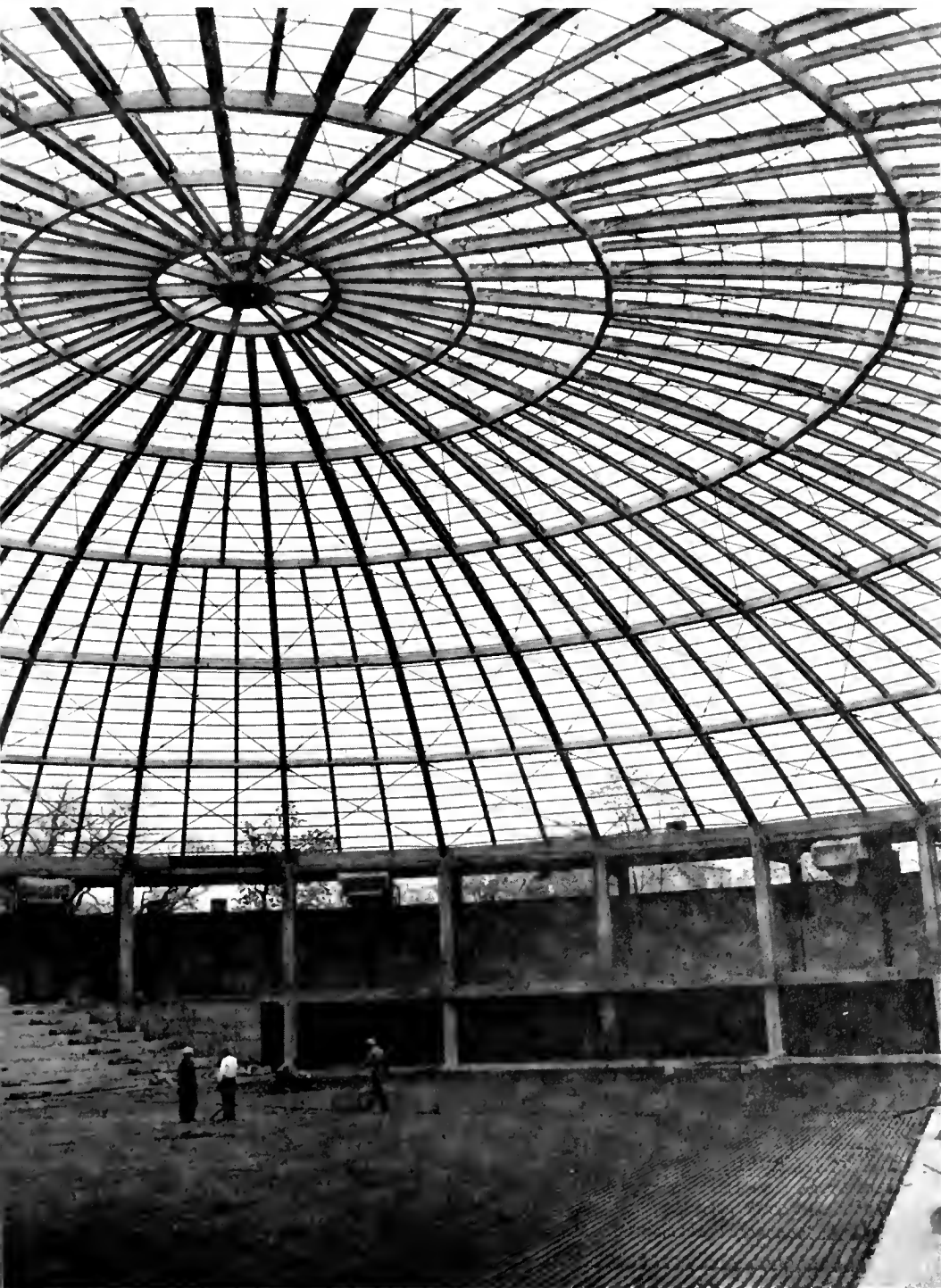
LAYING 10 MILES of brine pipe was only one of many spectacular construction operations.
