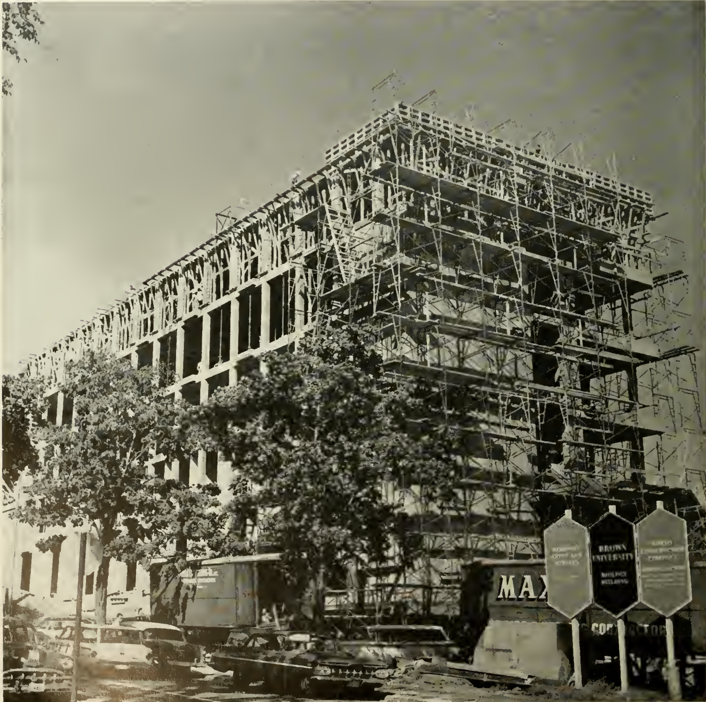
BROWN'S NEW BIOLOGY BUILDING at Brown and Waterman Sts. was approaching its full height when this photo was taken earlier in the fall.
