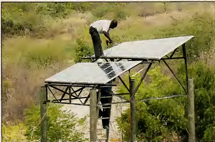
STANDING over solar panels, a worker installs the solar modules that power the water pump. Frank Viscomi, a university engineer, helped install the pump which provided over 5,000 gallons of water on a daily basis. Photo courtesy of Mary Tacy.
