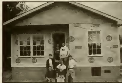
A few weeks before the house's dedication, members of Habitat and the Greek community display their progress. The house was built to be wheelchair-accessible for Isaac Carter, one of the new house's residents. ■ Photo by Todd Grogan
