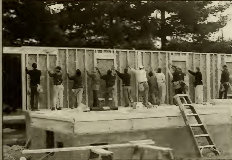
Students work with community volunteers to erect the first wall at Habitat for Humanity's house in Grottoes. The construction was supervised by volunteers from Nielsen Construction Co. and was helped by the campus Greek community. ■ Photo c/o Karen Calkins
