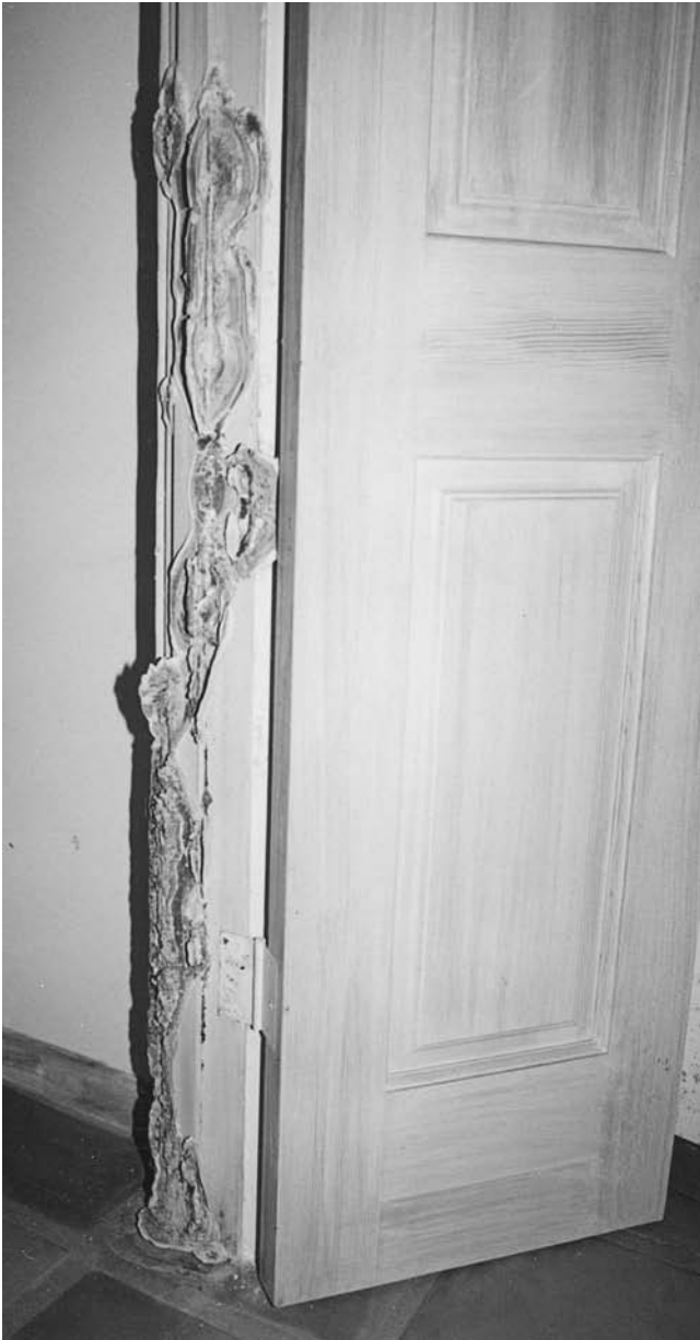
Fig. 14.1. Basidiomes of Meruliporia incrassata on door frame in Californian home damaged by dry rot. Photograph courtesy of Luis De La Cruz (De La Cruz Wood Preservation Services, Van Nuys, CA).
